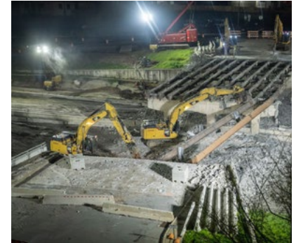
I-30 reconstruction continues in downtown Little Rock. Demolition of the 6 th Street overpass. Photo: Kelie Wylie and ARDOT.
