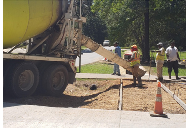
Installation and maintenance of sidewalks, such as these in Shannon Hills, are the responsibility of local jurisdictions.
