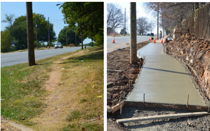
Metroplan and the city of Little Rock worked together to replace a dirt path with a sidewalk to better connect Our House with the nearest bus stop.
