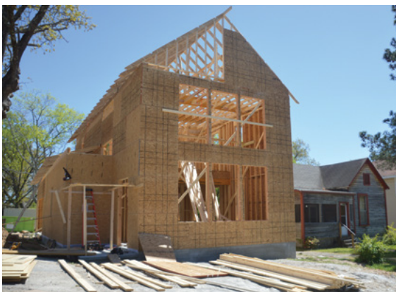
A single-family home under construction by Common Ground Development Co. in the Pettaway neighborhood.
