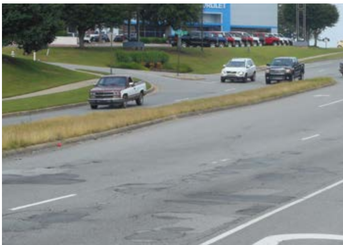
Chenal Parkway was built a quarter-century ago by developers. Now Little Rock’s responsibility, it is showing its age.
