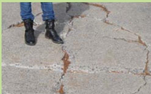
Cracking pavement is surpassing rebuild efforts all across suburban America.
